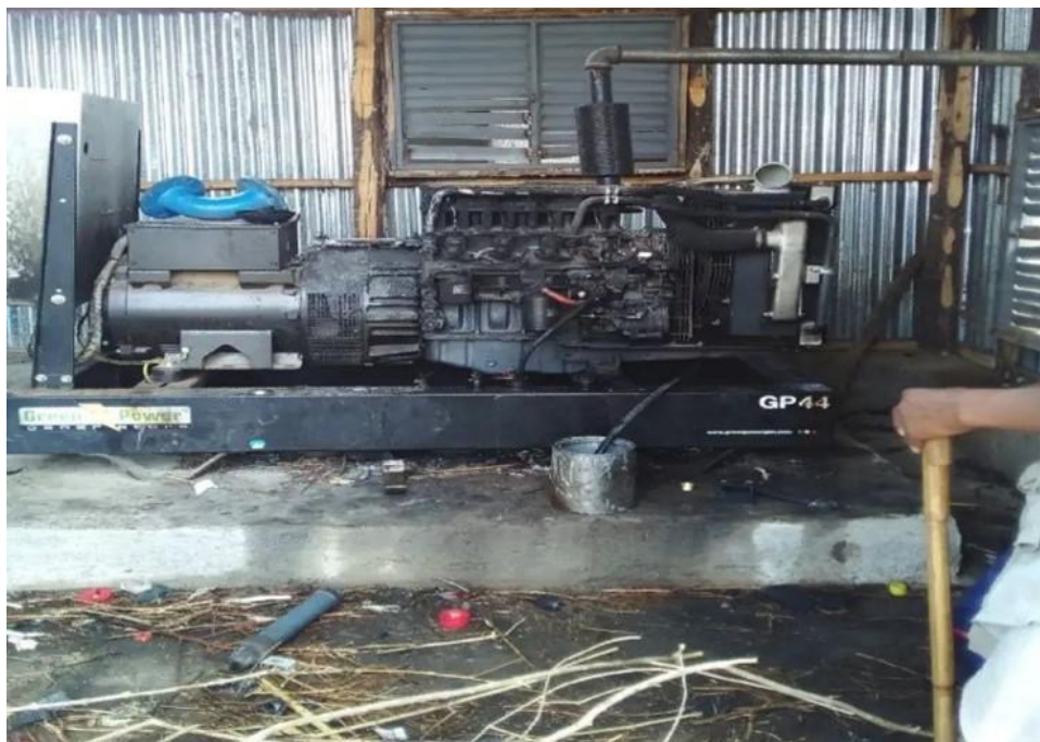
Figure 9: power generator burned in Haile Mariam Kebele (Antsokiyana Gemza Woreda).
