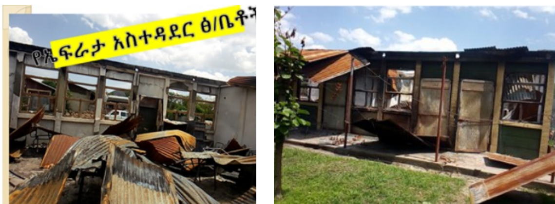
Post-attack situation of Efratana Gidim Woreda Administration Ataye Town Administration Offices 2/2
